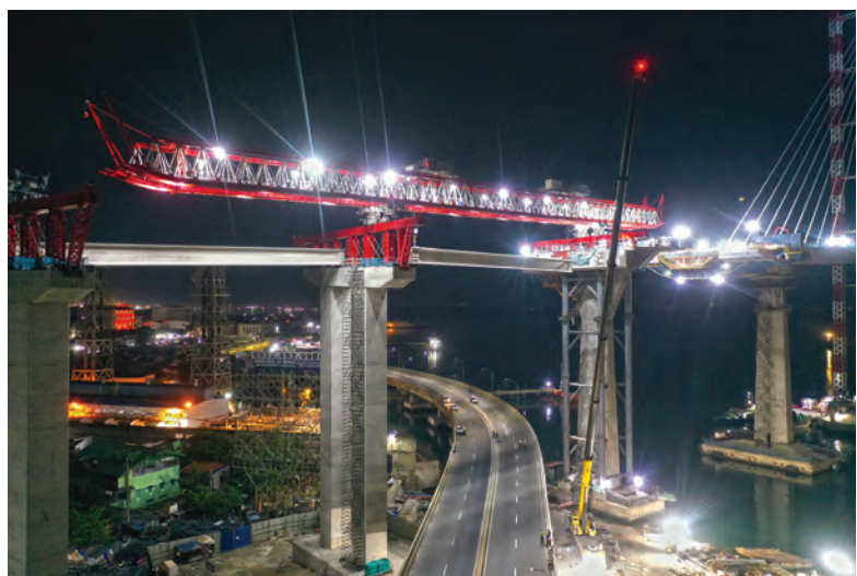
IMAGES ON THIS PAGE: CCLEX provides two lanes in each direction that will offer a safe, quick and scenic passage for approximately 50,000 vehicles daily. It has a design speed of 80 km/hr and a navigational clearance (height) of 51 m to allow large vessels to pass underneath the bridge.
